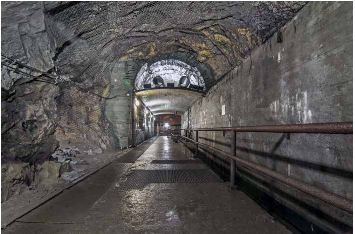
Main gallery at Rzezka showing partially completed concrete lining. The roughness of the original excavation must have massively increased the volume of concrete needed. The smaller higher level passage would have been used for ventilation and other services. Photo Chris Wilkins
